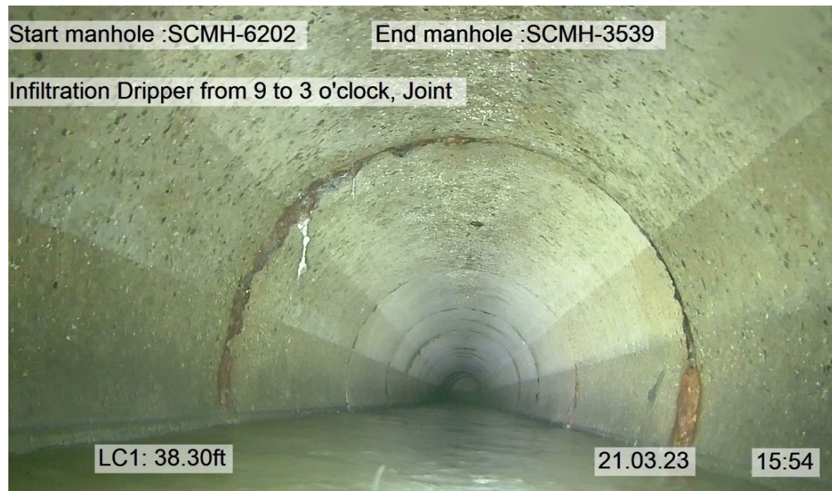
Image at 38.30' shows infiltration.
