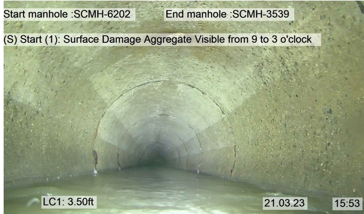
Image at 3.50' shows aggregate visible.
