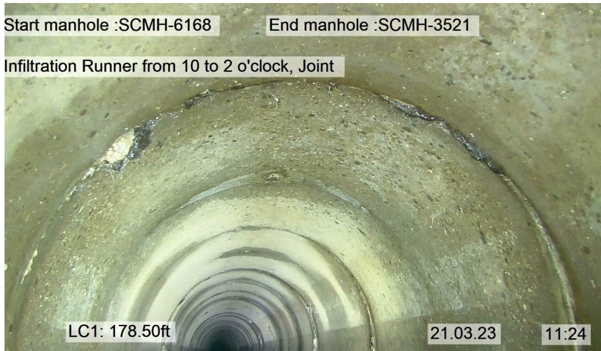
Image at 178.50 shows infiltration.
