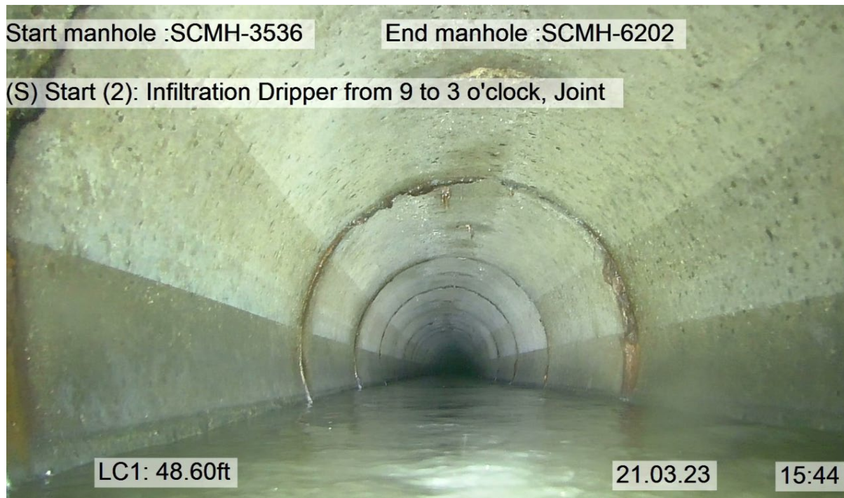
Image at 48.60' shows infiltration.
