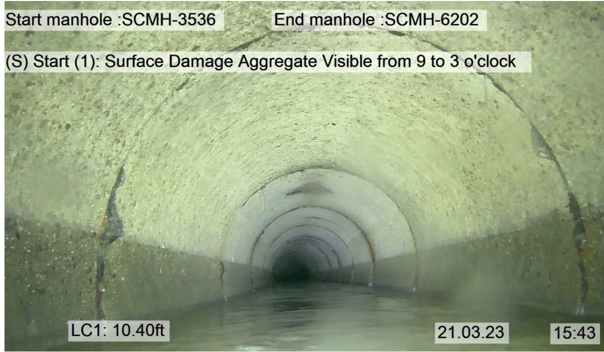
Image at 10.40' shows aggregate visible.
